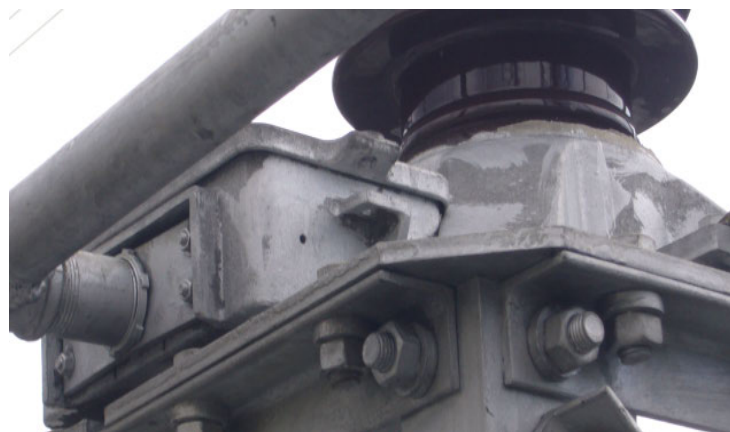
Zapote – Secondary terminal box has no seal
