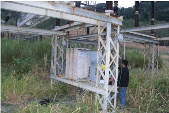
AFAB – Excessive vegetation growth
