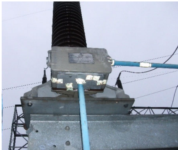
Petron – Joints of all conduits are sealed
