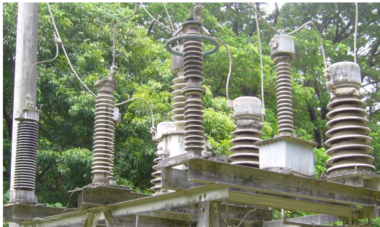
Northern Cement Corp. – Heavily contaminated bushings of CT and PT
