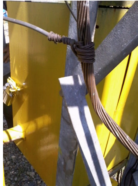
INECO – Non-standard Ground Connection (spliced; poor contact)
