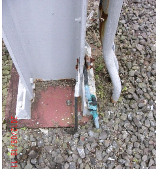
Makban – Corroded ground with poor connector
