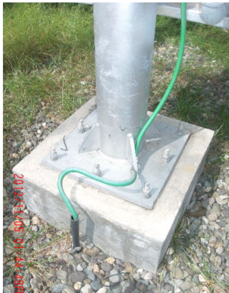
KEPCO – Ground down conductor (jacketed, green, big loop, with protection at grade level)
