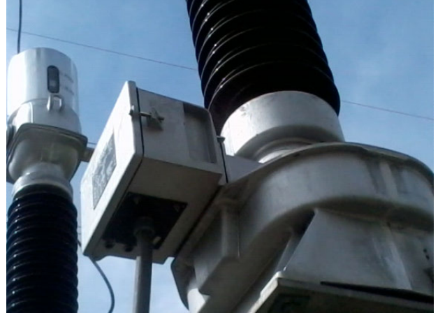
KEPCO – Secondary terminal box has no provision for seals
