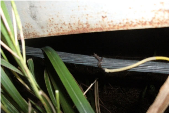
AFAB – Poor grounding connection
