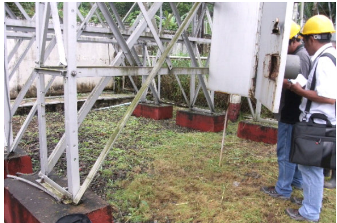
PUD – With vegetation growth (grass was cleaned only hours before inspection)
