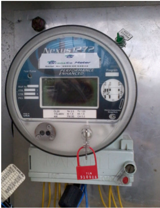
Masinloc – Blackened meter display
