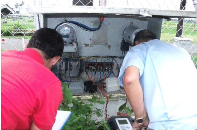
UPLB – Dilapidated meter enclosure
