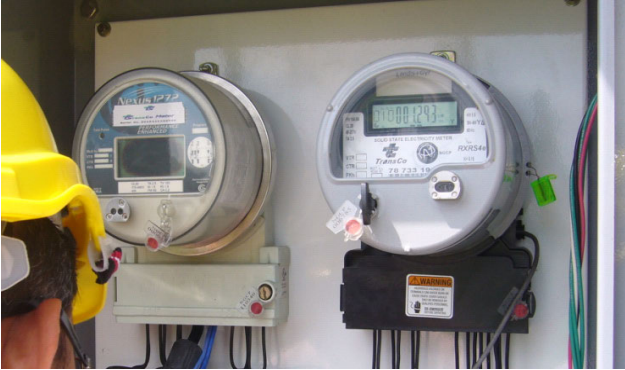
Angeles Electric – Blackened meter display
