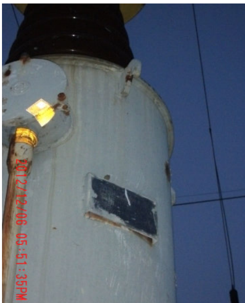
AFAB – Sticker seal on secondary terminal box
