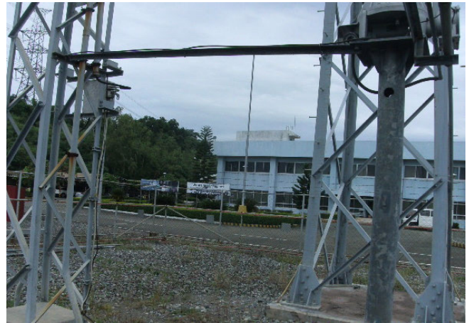
Masinloc – Overhead ground interconnection
