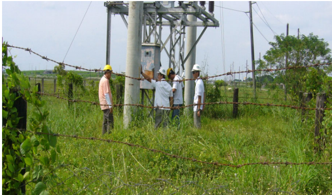
Clark Electric Distribution Corp – Heavy vegetation
