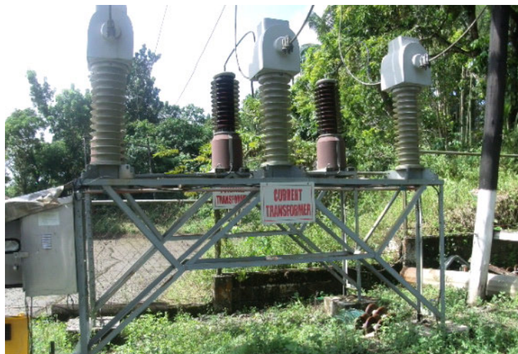
AKELCO – Heavy vegetation with debris
