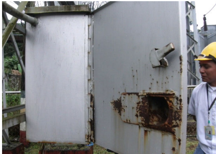
PUD – Meter enclosure is heavily corroded
