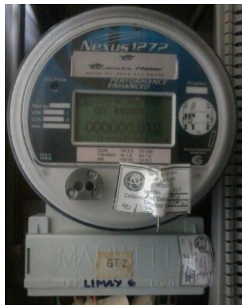
Bataan CCPP – Sticker seal used
