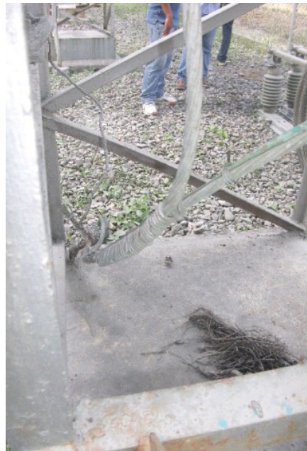
Carmen Copper - Ground connection by splicing (instead of exothermic or compression method)
