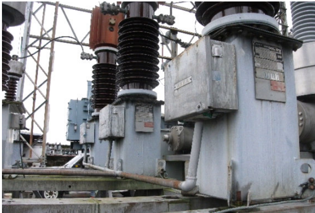
PELCO II Guagua – Corroded tank and structure
