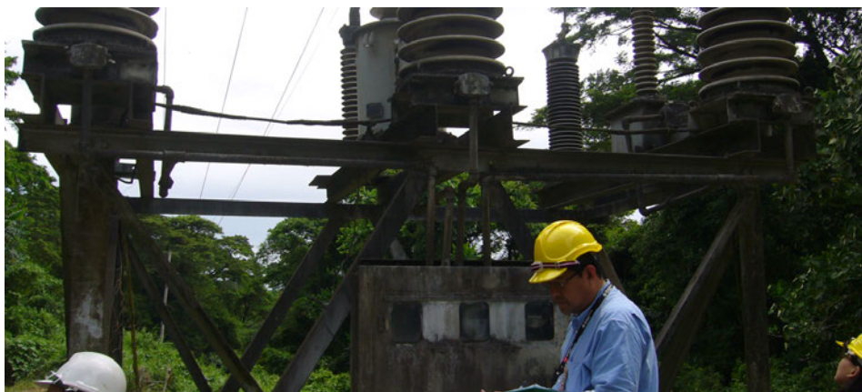
Northern Cement – No perimeter protection (fence or gate)
