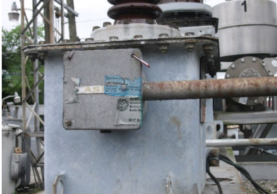
PELCO II Guagua – Mechanical and sticker seals combined
