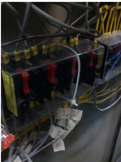
CBK – No seal; only cable tie was used
